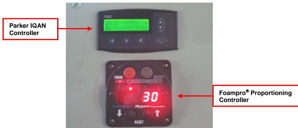
Figure 3.8.3: UHP P-19 IQAN control monitor along with the foam proportioning controller.
