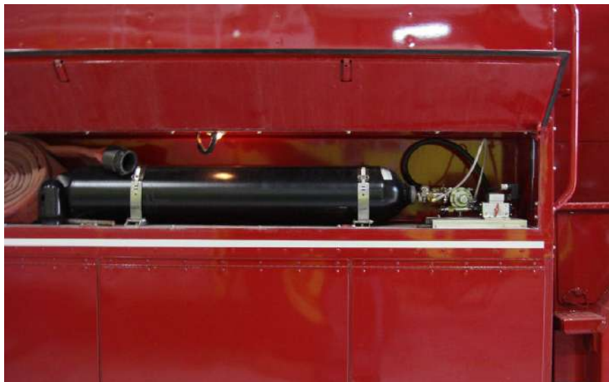
Figure 3.6.2: The high pressure nitrogen tank used to pressurize the dry chemical storage tank.
