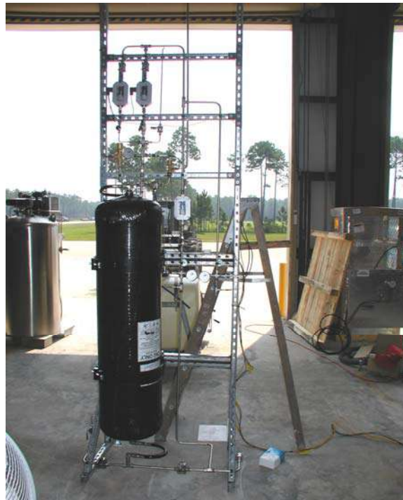
Figure 2.1.2: Liquid/supercritical CO 2 injection system.
